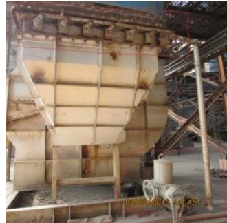
Before: All bag filter fans in DOL Operation
