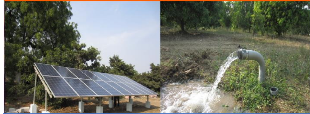
Solar Water Pump at Mango Garden
