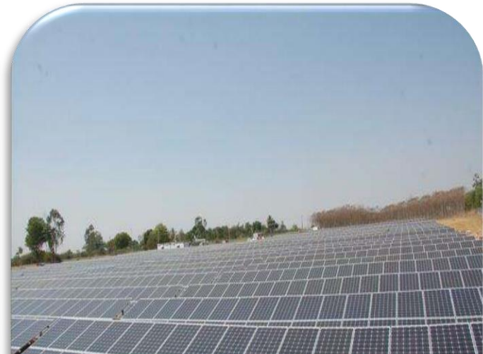
SOLAR POWER PLANT, MUKTYALA – 1.15 MW
