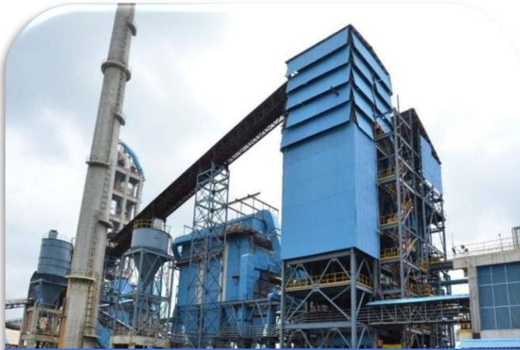
THERMAL POWER PLANT, MUKTYALA – 1X18 MW
